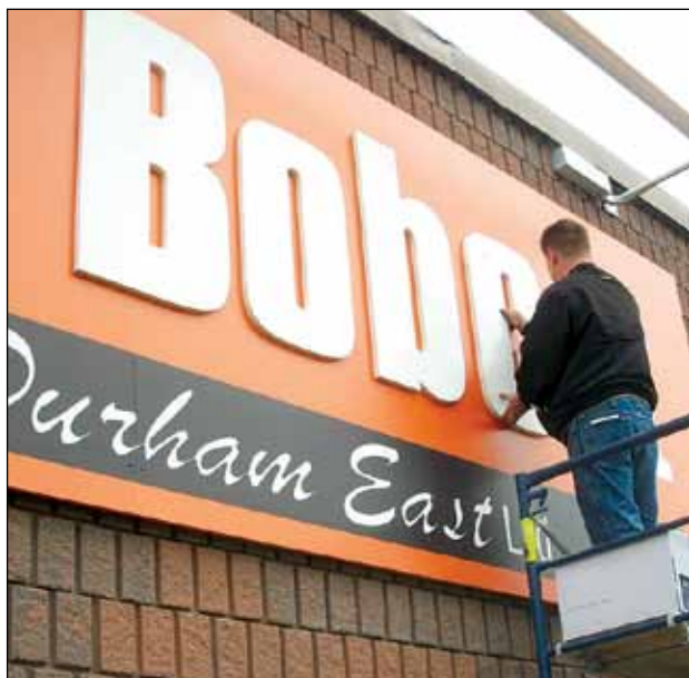
James Printing & Signs employee, Vance Sutherland, installs cut letters onto pre-printed board for Bobcat of Durham East. Nice sign Jeff!
